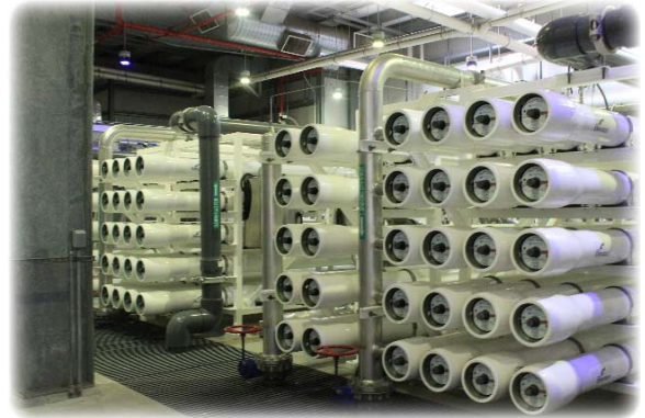
Filtration System at the CDA II Treatment Facility
